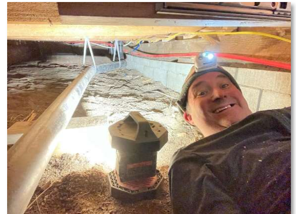
plumbing under the bunkhouse
